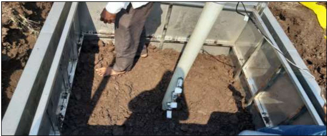
Plate 10. Layer wise soil refilling& compaction and sensor installation in the inner tank of Lysimeter
