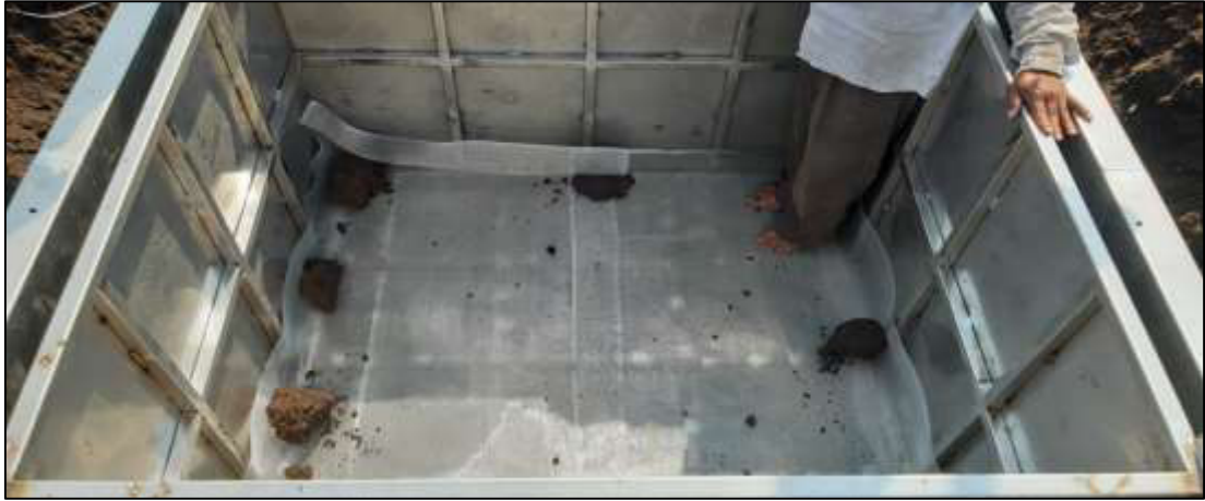
Plate9. Placing of mesh at the bottom of inner tank to prevent washing out of soil through drain
